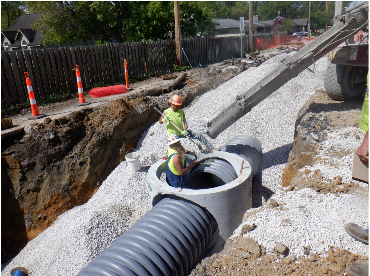
(BBI pouring concrete collars for 36" storm sewer pipe at Str. #136 along Walnut Street.)
