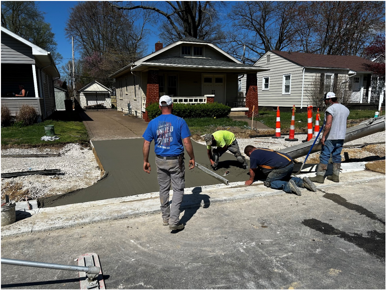
(BBI pouring exposed aggregate drive along Walnut Street between Weinbach Avenue and Boeke Road.)
