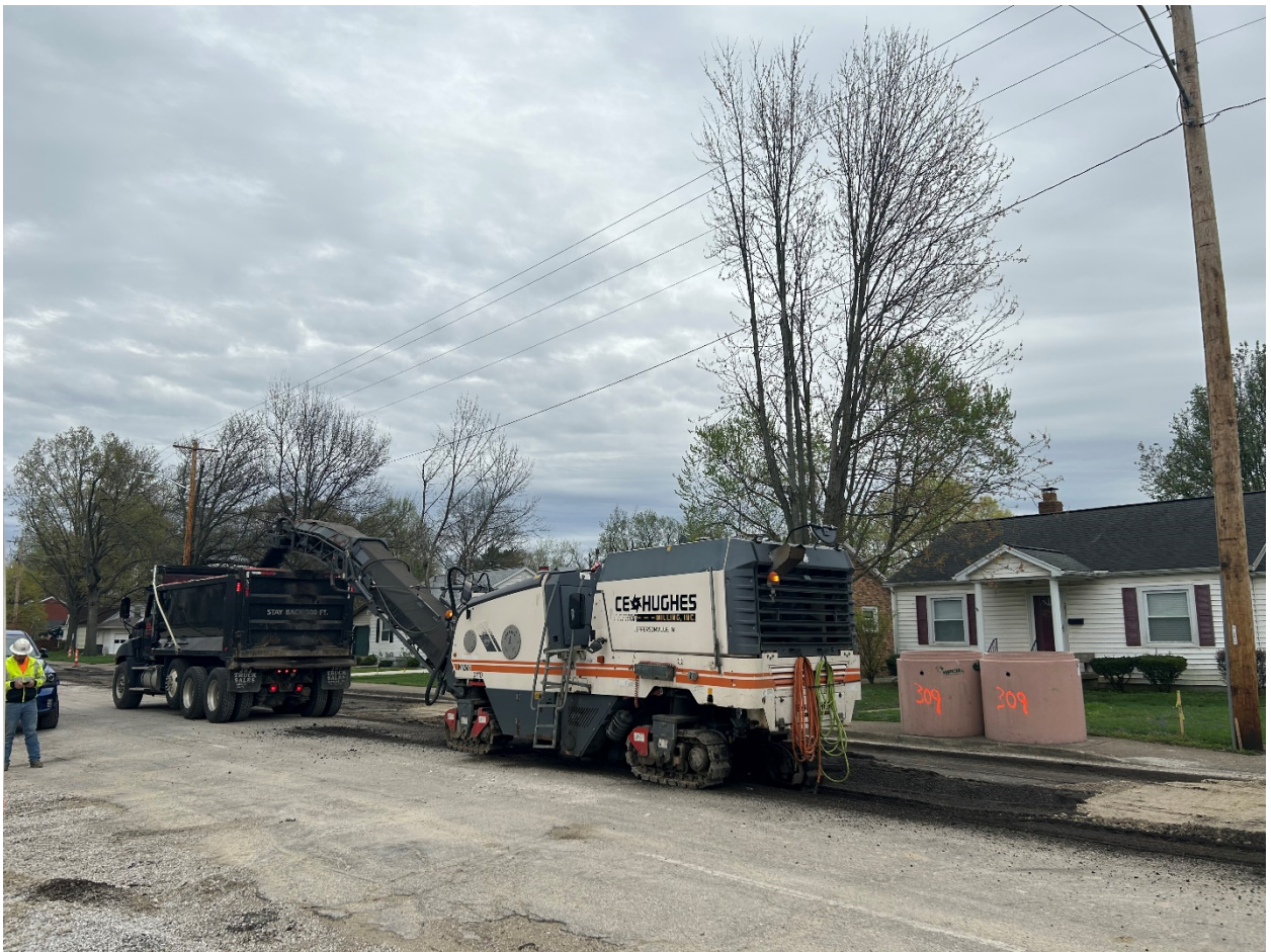
(CE Hughes milling two lanes on the south side of Walnut Street from Boeke Road to Vann Avenue.)
