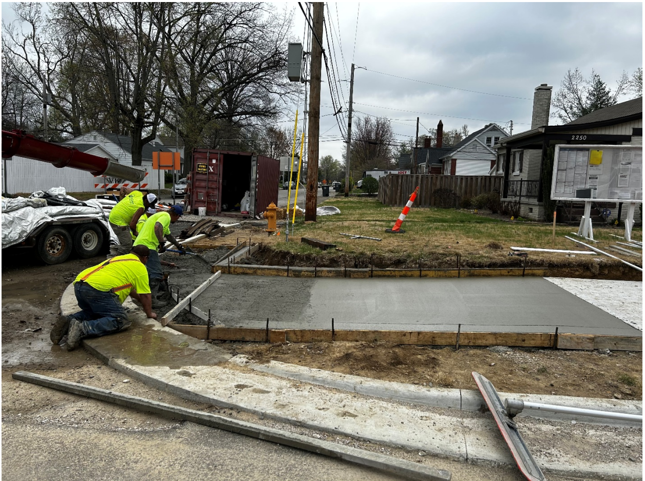
(BBI finishing the curb ramp for the multi-use trail at Fairlawn Avenue and Walnut Street.)
