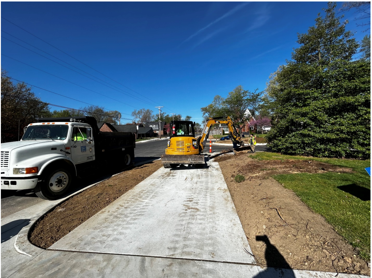
(BBI continuing to grade backslopes along multi-use trail for Walnut Street at Alvord Blvd.)
