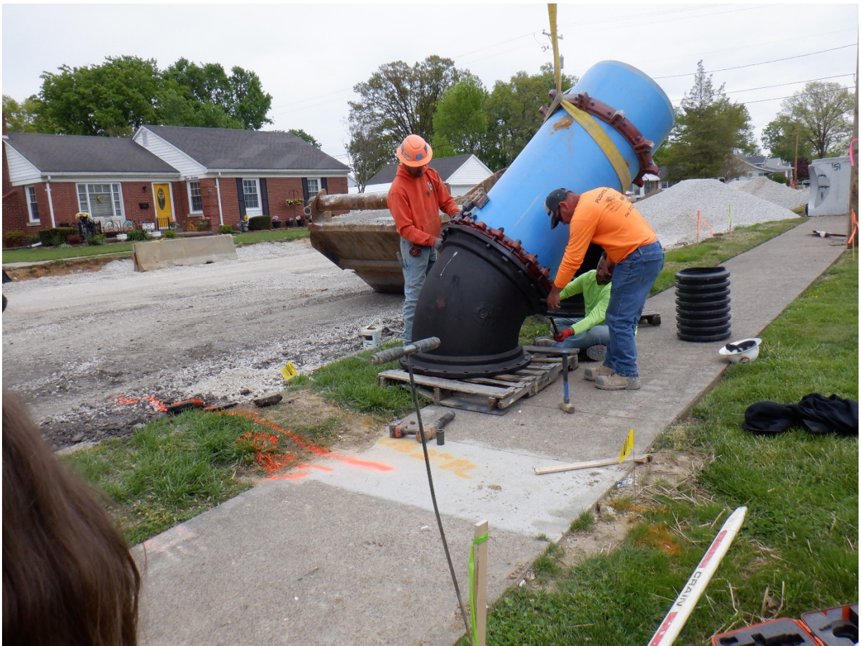
(BBI bolting on 45 degree horizontal bend onto 30" force main before installing along Walnut Street.)
